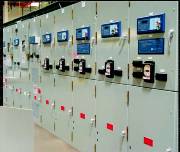
Medium Voltage Switchgear
