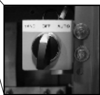
Selector switch operator for contactor operation
